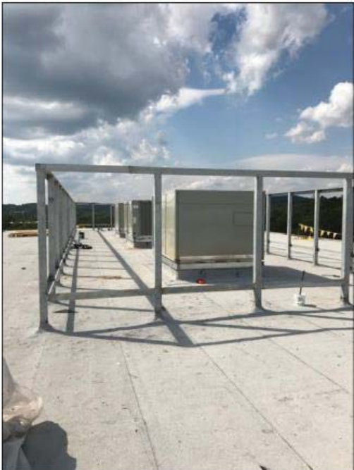
Roof Top Units
